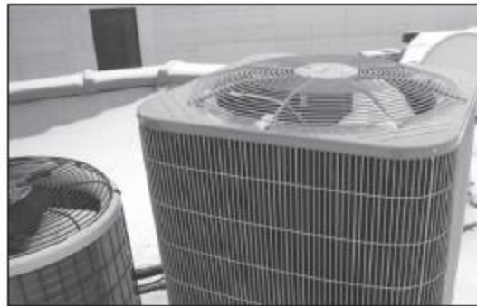
Air conditioning systems
